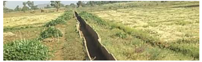
Figure 5. Tertiary canal degradation
