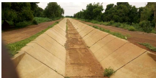
Figure 4. Primary canal silted up and covered in grass during low water periods
