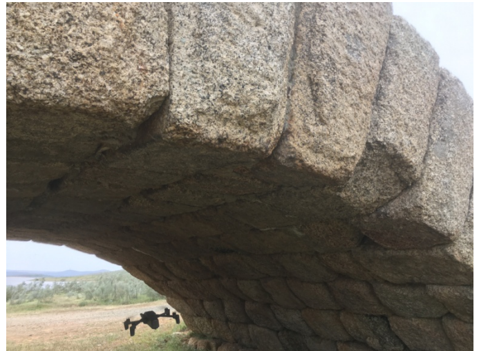
Fig. 3. Quadcopter drone circulating inside the first vault of the Roman Bridge of Alconetar (Spain), for its intrados inspection (photo by the author)
