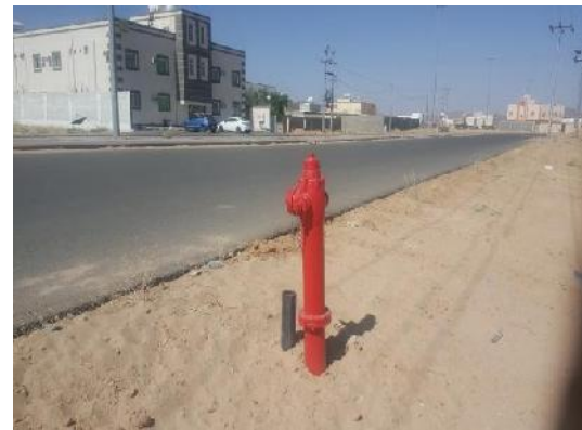
Figure 22. Red street hydrant (13)
