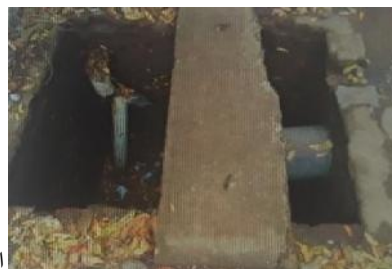
Figure 36. Street trenches are not all covered (34)
