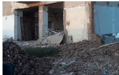
Figure 8. Debris and rubbles in streets (13)
