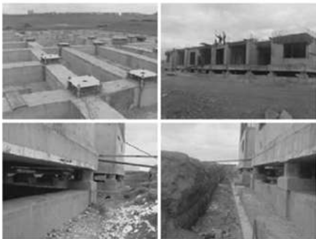
Fig. 3.5. Seismic isolators used in Parand
